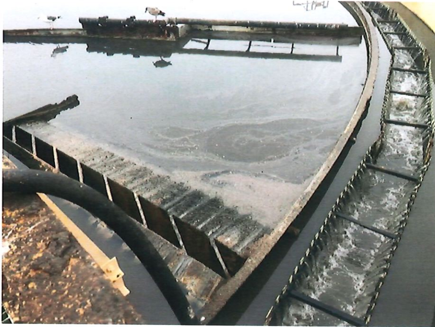
Figure 6: Scraping SKIMMER mechanism of primary clarifier.
