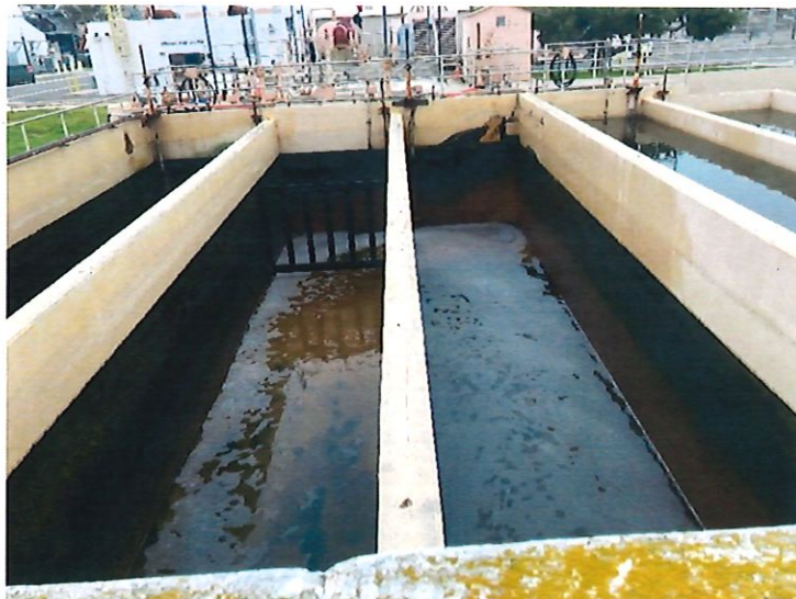
Figure 13: Chlorine contact basin used to promote contact time between disinfectant and pathogens.
