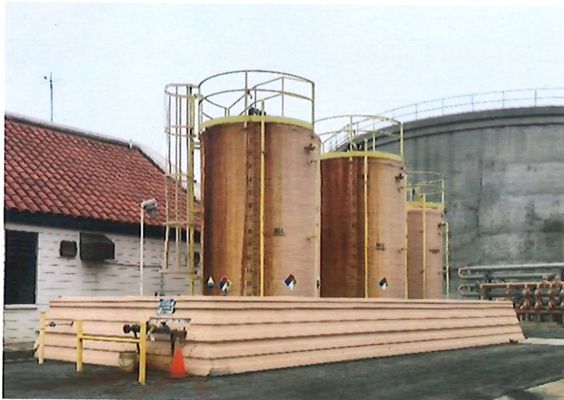
Figure 7: Ferric chloride storage onsite.
