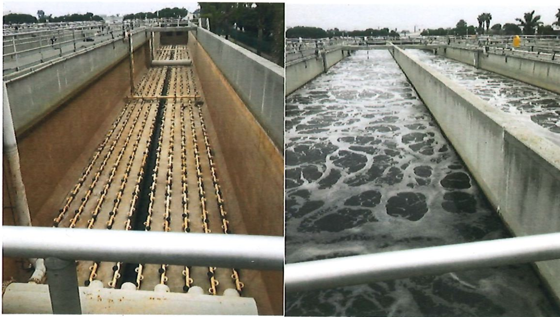
Figure 8: Activated sludge tanks, empty (left) and full (right).
