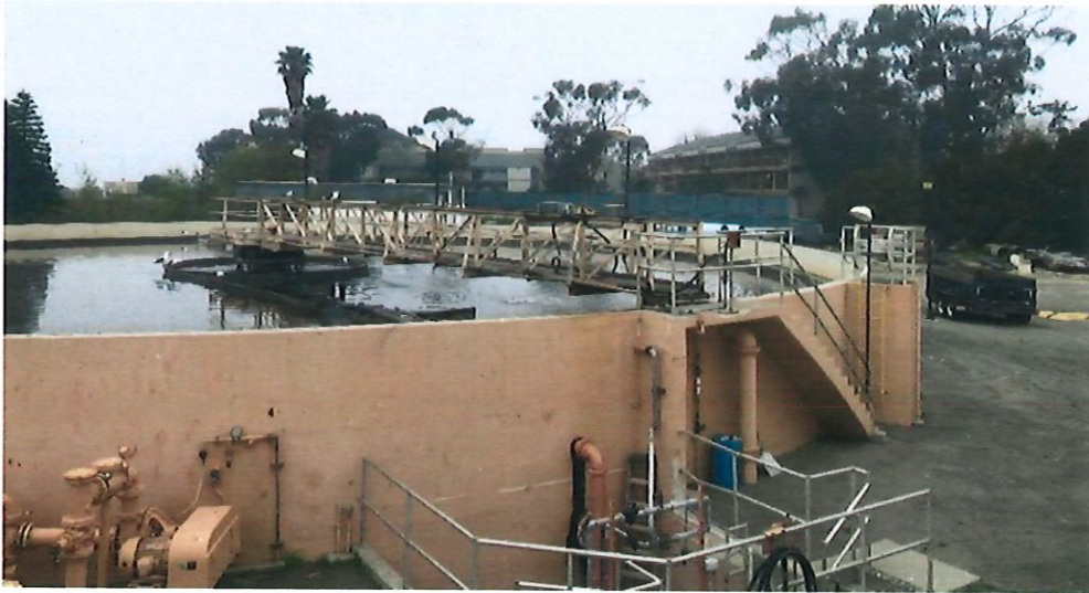
Figure 5: One of four primary clarifiers onsite.
