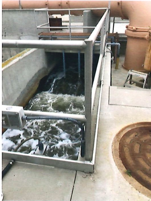
Figure 11: Sodium hypochlorite injection following secondary sedimentation.
