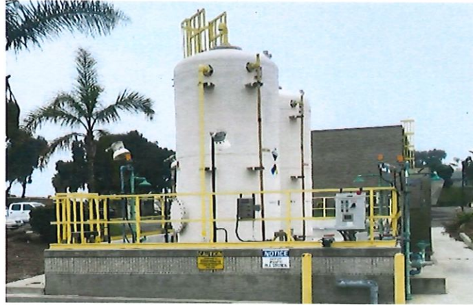
Figure 14: Sodium bisulfite storage and filling station.
