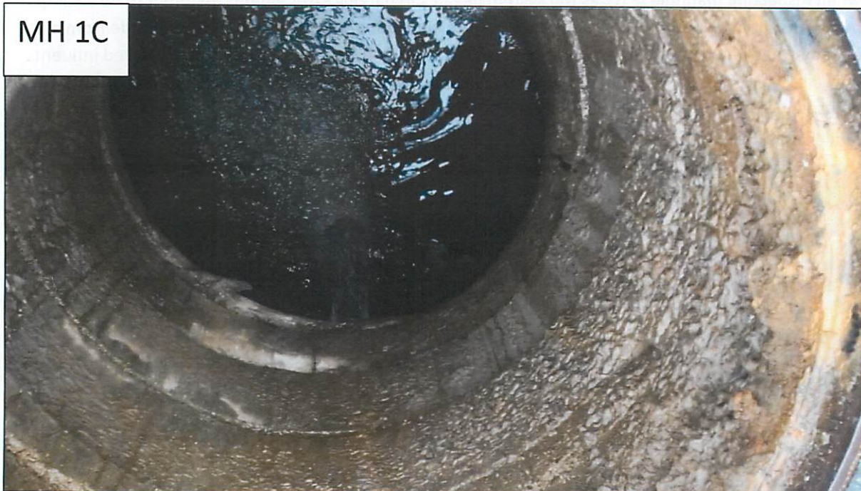
Figure 21. Observed surcharging in Manhole IP6.
