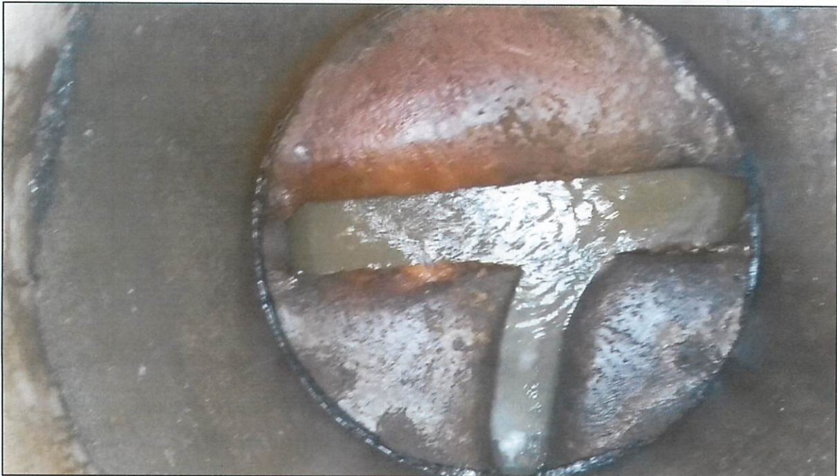
Figure 15. Observed constant groundwater infiltration through crack in Manhole IP6.
