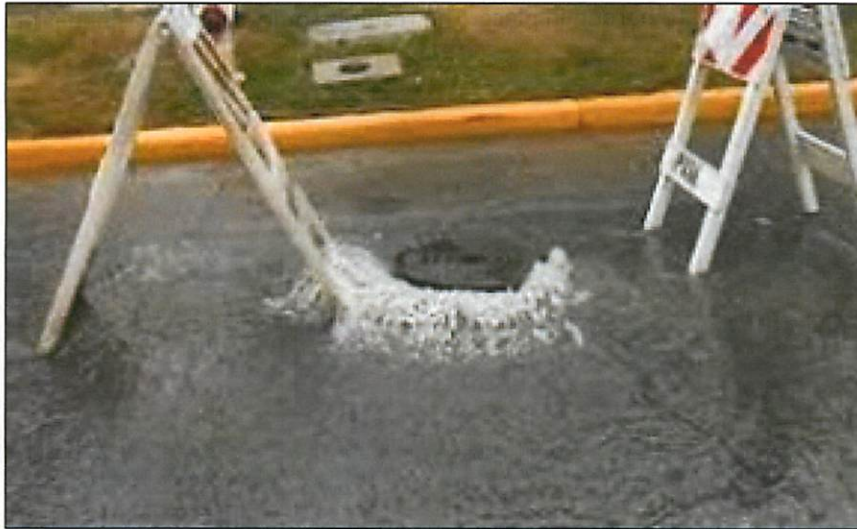
Figure 5. A sanitary sewer overflow occurring in Arcata (City of Arcata).
